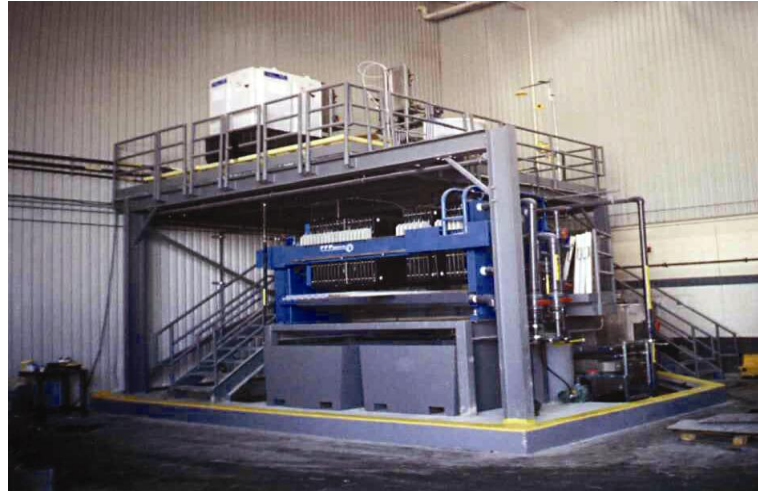
Dissolved Air Flotation (DAF) with Recycle Skid 30ft3 Filterpress with servo-assist plate shifter Control Panel with PLC.
