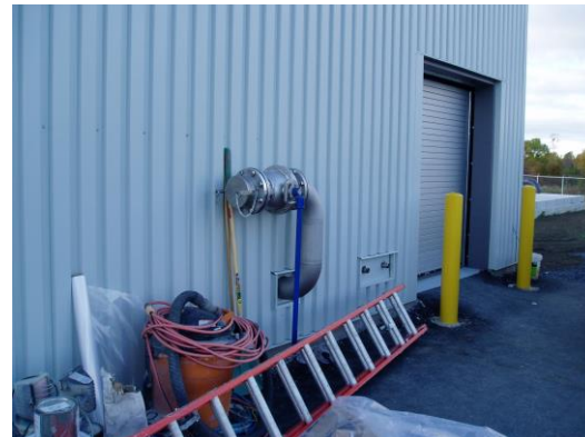
Outside Hose Connection
