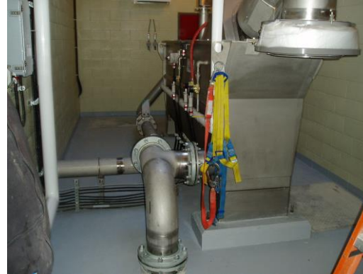
Continuous Solids Bagging Unit
